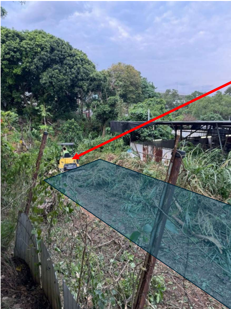
A small Bulldozer is used to clear the vegetation on the stream
